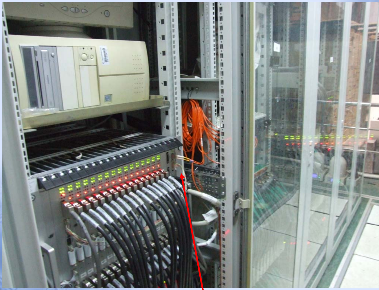
TCBA: EMC preprocessor and transmitter
